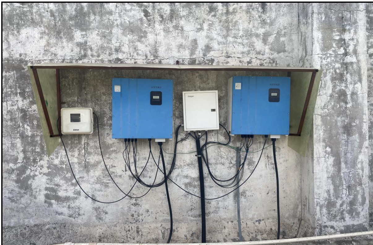
Figure 2.6:- Solar Plant 480 KWp and Inverter System
