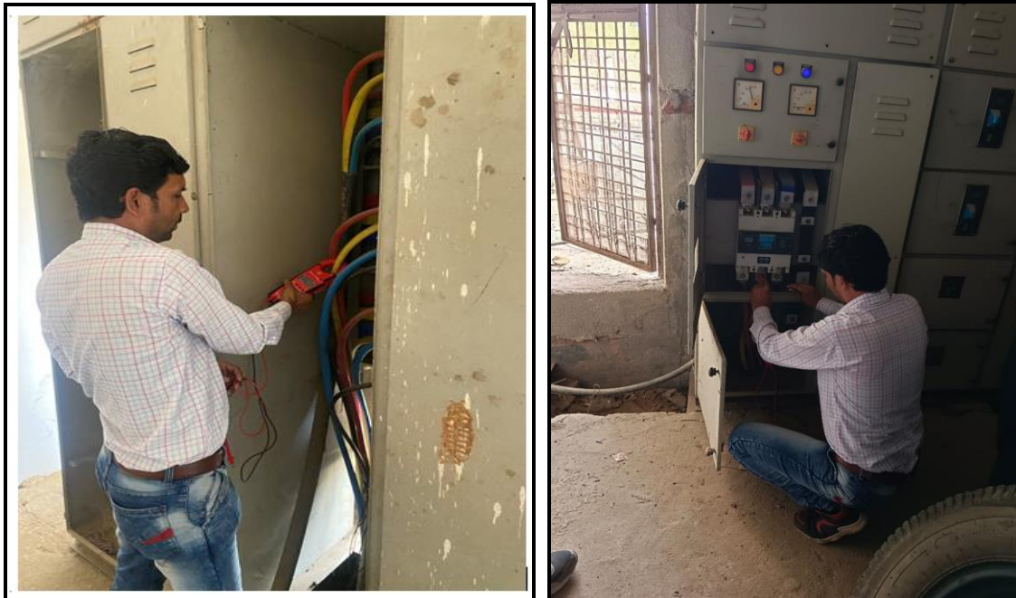
Figure 3.7:- On-site power measurement Dated 16/05/2022
