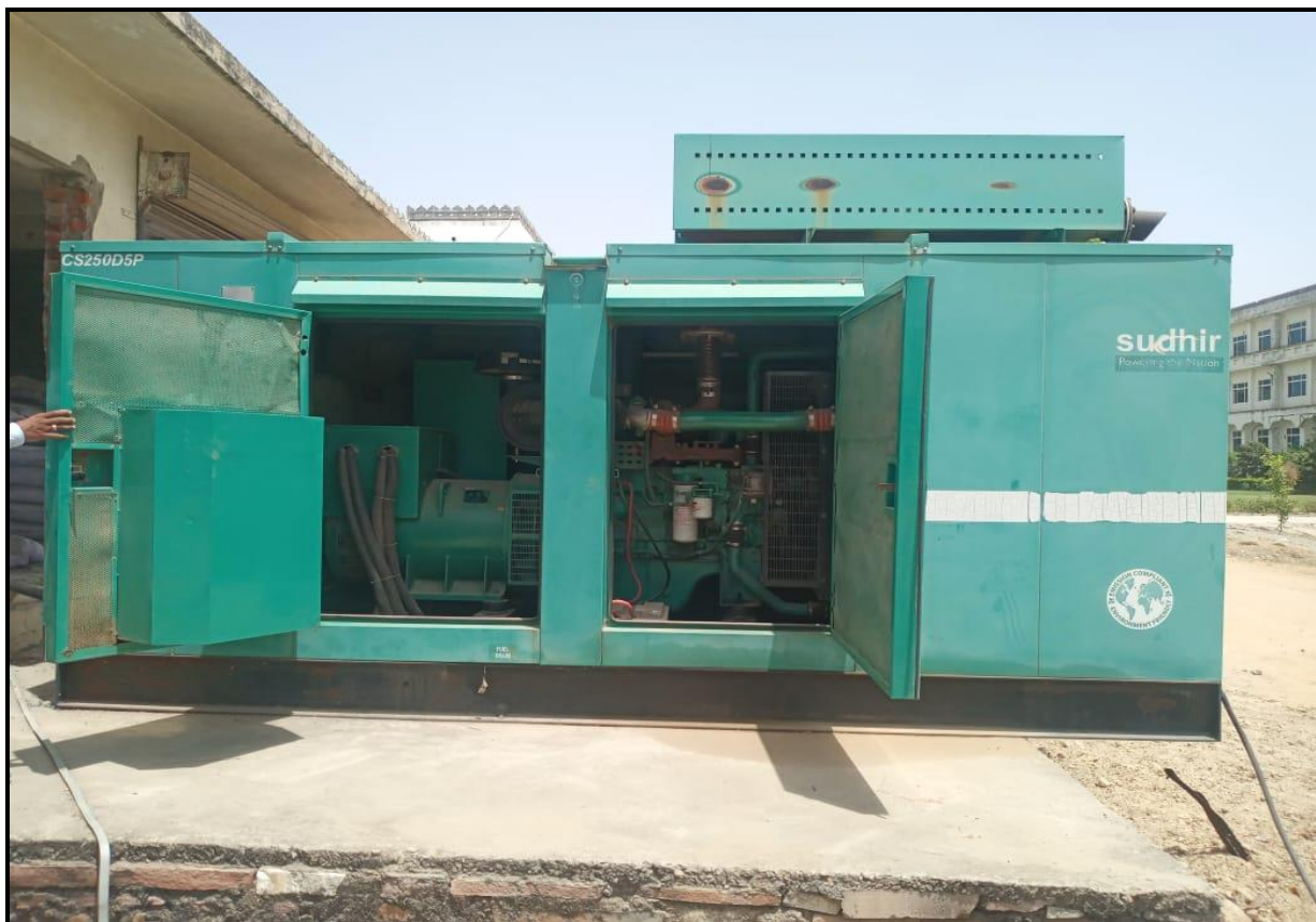
Figure 2.4:- DG set in Power House
