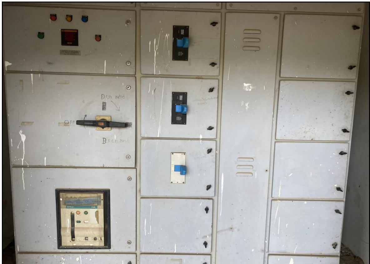
Figure 2.5 Capacitor bank on main panel
